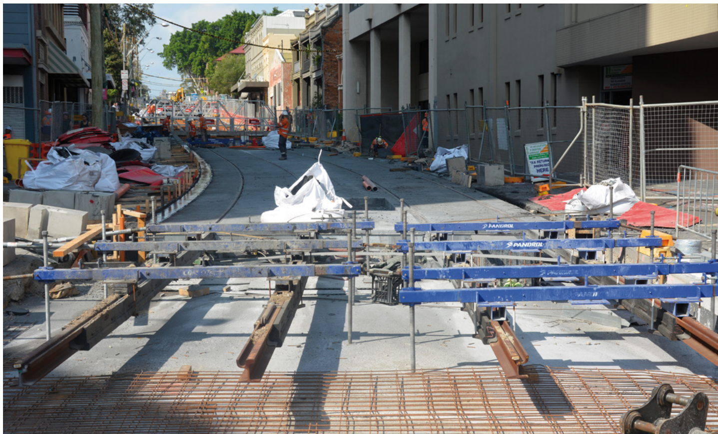
A section of partially complete light rail in Devonshire Street, Surry Hills, just east of Elizabeth Street, where there are also sections with no track laid and excavations for track are yet to be commenced on Thursday 26 April. Diverting utility services still appears to be delaying works in a similar manner to that still delaying track laying in parts of George Street. Shane O'Neil
